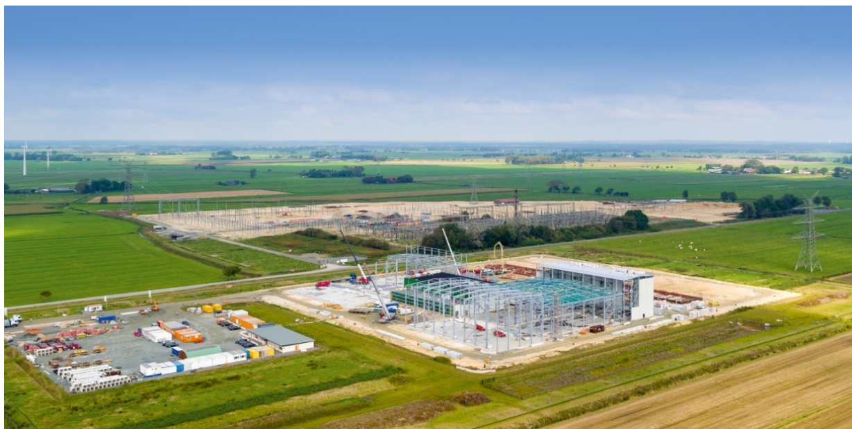
The NordLink converter construction site at Wilster (in the background: Wilster West transformer substation) in September 2017
